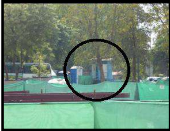
Figure 2.7. Mobile Toilets Arrangements
