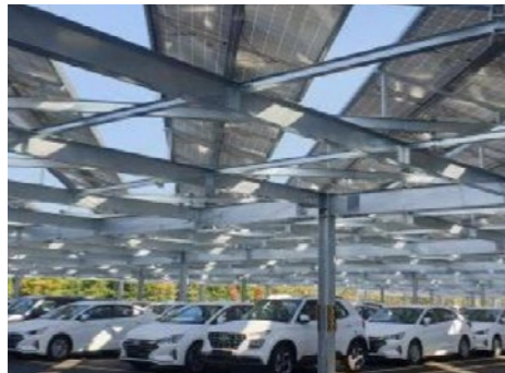
A photovoltaic power generation facility in the parking lot of the Ulsan Plant's driving test site
