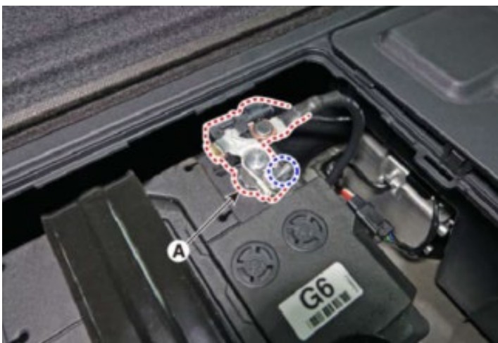
4-2. Turn the ignition switch OFF and disconnect the auxiliary 12 Volt battery negative (-) terminal (A).
